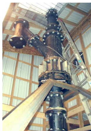
The gasifier being developed by Taylor Energy and the Western Research Institute.
