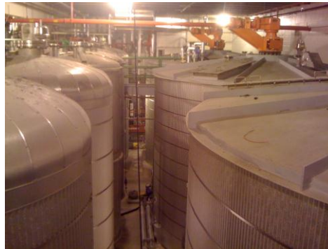
35,000-gallon hydrolysis reactors
