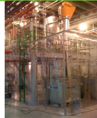
10 T/D pre-treatment skid
