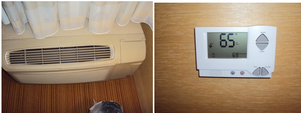
Figure 11. Photograph of a Carrier PTAC unit and Telkonet OBC thermostat at Courtyard Los Angeles Torrance/South Bay
