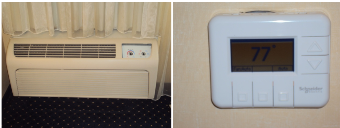
Figure 19. Photograph of an Amana PTHP unit and Schneider Electric OBC Thermostat at Courtyard Gaithersburg Washingtonian Center.
