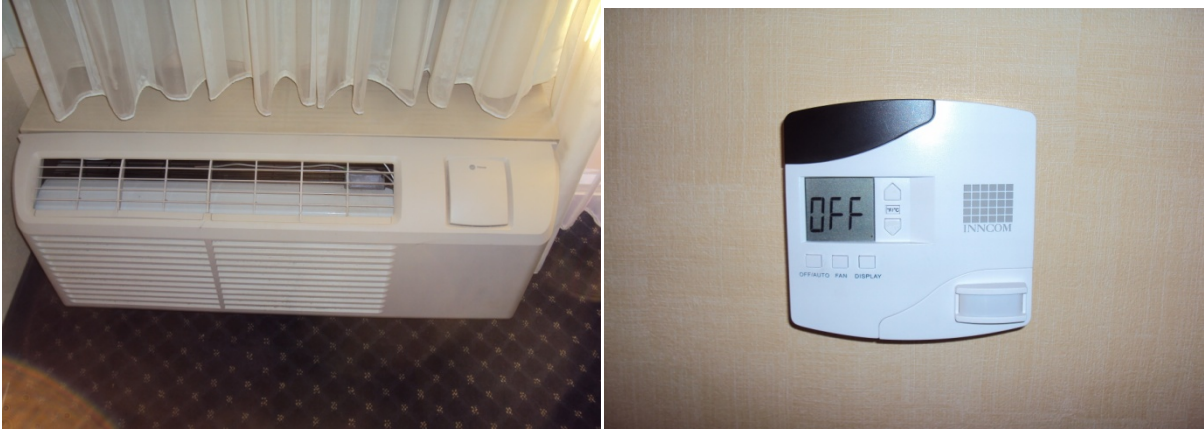
Figure 8. Photograph of a Trane PTAC unit and Inncom OBC thermostat at the Courtyard Dallas Richardson at Spring Valley.
