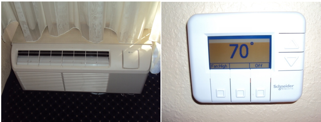
Figure 5. Photograph of a Trane PTAC unit and Schneider Electric OBC thermostat at Courtyard Dallas Addison/Midway
