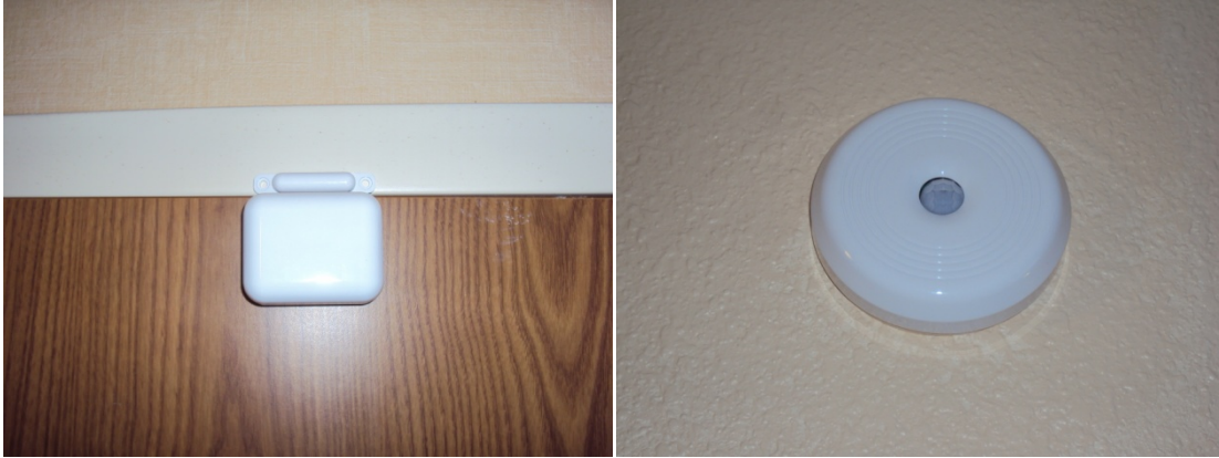
Figure 6. Photograph of a Schneider Electric Wireless Door Switch and wireless occupancy-sensor at Courtyard Dallas Addison/Midway.
