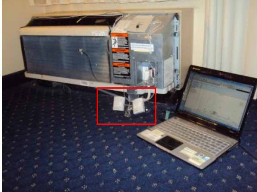
Figure 1. Photograph of a PTAC (exterior casing removed) showing two data loggers (inside highlighted box) at the Courtyard Dallas Richardson at Spring Valley, Richardson, Texas.
