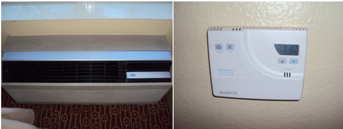
Figure 13. Photograph of a Carrier PTAC unit and Onity OBC thermostat at TownePlace Suites Los Angeles LAX/Manhattan Beach
