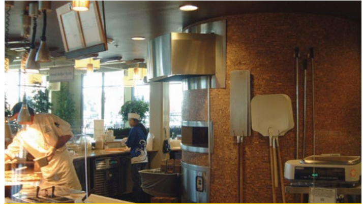
The commercial kitchen at the Raleigh Whole Foods Market was a prime target for efficiency improvement.
