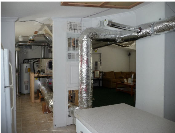
Figure 2-3. System air handling unit shown on the left side of the utility room area, with the main duct and branch in the kitchen
