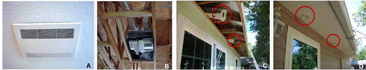
Figure 3-7. Ceiling-mounted energy recovery ventilator (A,B) installed in the main body with attic-mounted supply and exhaust ducts (B,C) terminating in soffit-mounted registers (D)
