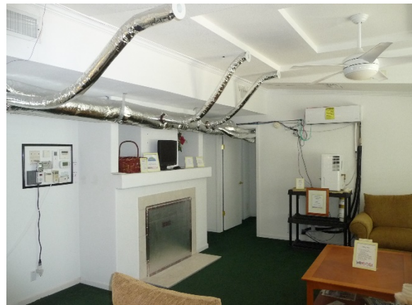
Figure 2-4. Main 8-inch duct with 2-inch ducts shown in living room area. A dehumidifier is against the wall below the ductless minisplit.
