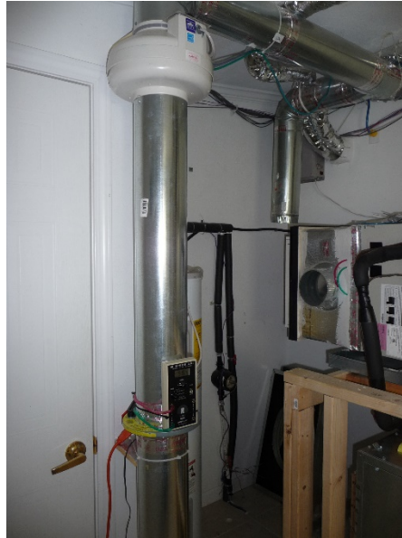
Figure 2-5. Mechanical ventilation supplied to the utility room
