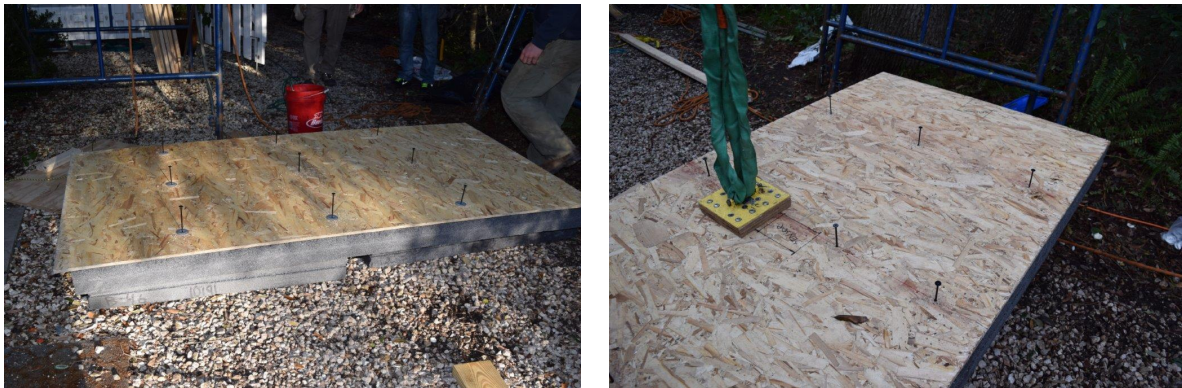
Figure 38. Pre-installed screws (Note the sensor location marked on the OSB next to the cleat.)
