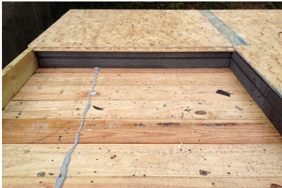
Figure 31. Oriented strand board surface spline and sealant at deck above rake wall
