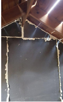
Figure 27. Rigid foam insulation at attic gable walls
