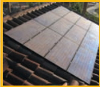
Solar electric panels mounted unobtrusively on the roof on the back side of the house.
