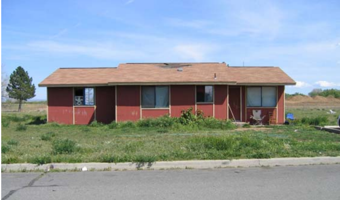
Figure 2. Another of the homes at Adam's View (shingles blown off roof)
