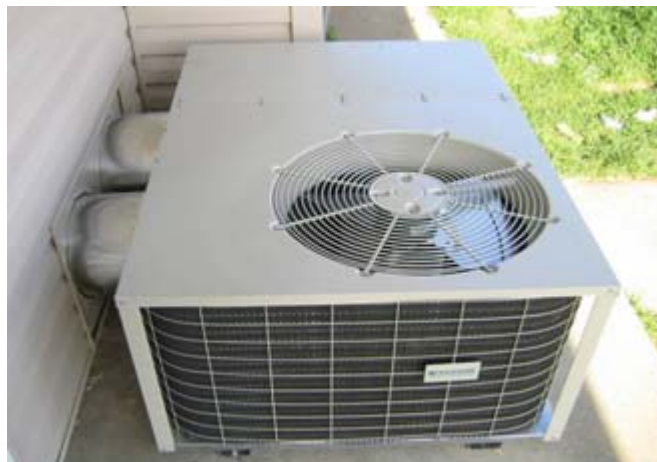
Figure 9. Packaged heat pump unit for house #303
