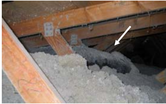
Figure 11. Ductwork partially buried in attic
