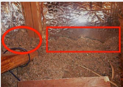
Figure 2. Duct section after insulation wrap has been installed. In the red rectangle, the foil facing will be tucked under and cellulose added. In the red circle, the foil facing is tucked under, and a small amount of cellulose insulation was added where the duct wrap meets the existing cellulose.
