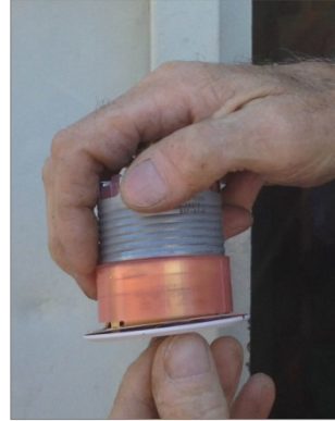
1/6-in. gap required by manufacturer that cannot be sealed
