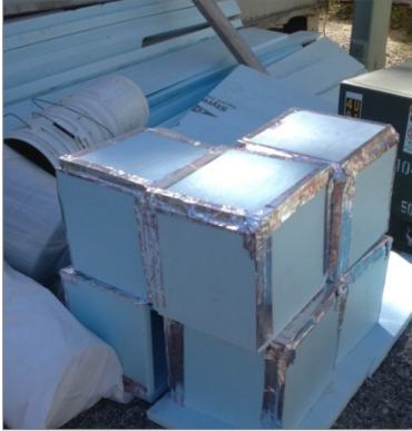
Insulated box for fire-suppression sprinklers used to help seal and separate from loose fill attic insulation
