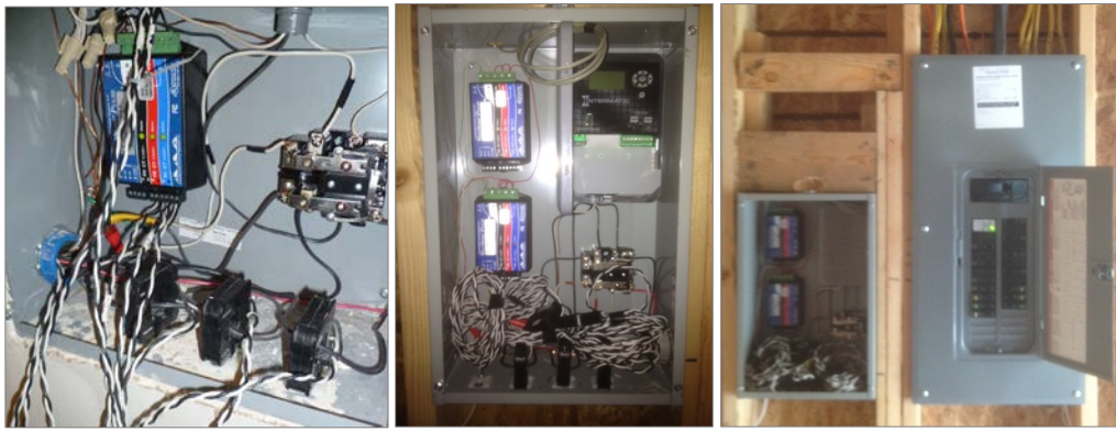
Figure 8. Panel containing time clock-contactors-CTs for switchback and monitoring
