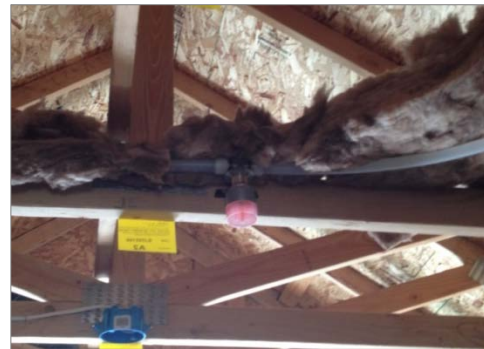
Sprinkler insulation freeze-protection tent over pipe
