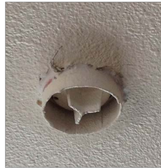
Installed sprinkler housing at dry wall stage prior to indoor head installed
