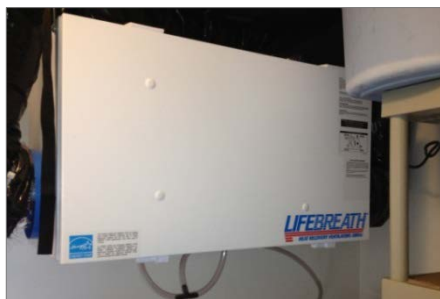
Limited access to changing filters (homeowner issues)
