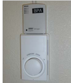
Figure 10. Indoor temperature/ RH data logger at zonal thermostat
