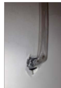
Kink in condensate drain (installer issues)
