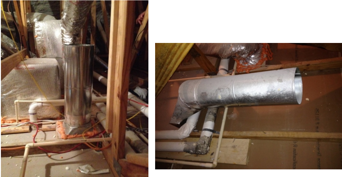
Figure 26. Vertical intake transfer duct connects to a vent in the mechanical closet’s ceiling (left); horizontal exhaust duct connects to 3-in. × 14-in. rectangular duct inside the wall cavity leading to the HPWH in closet (right).
