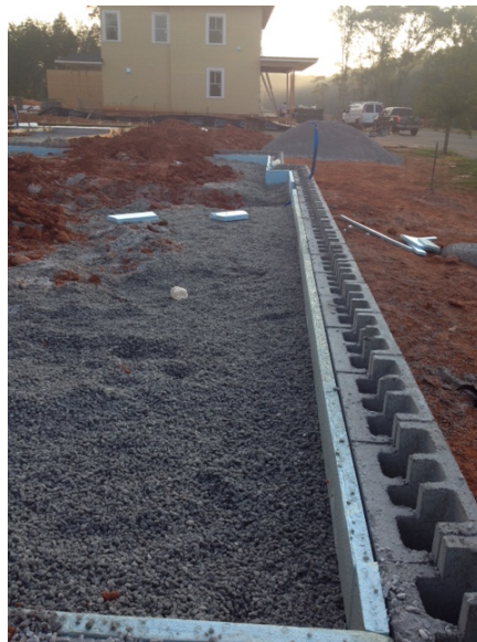
Figure 23. JMC elevated slab construction in progress showing gap insulation and stem wall
