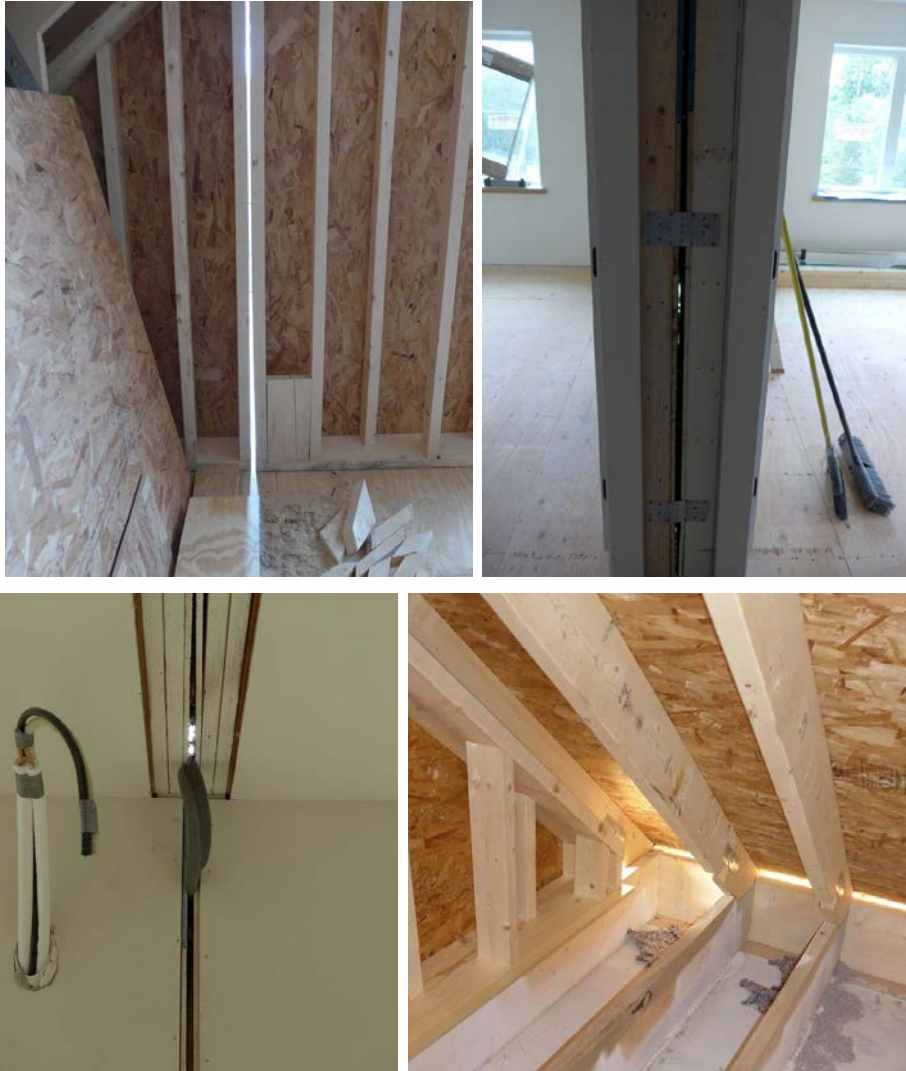
Figure 11. Gaps soon after set. Clockwise from top left: large gap in gable wall; daylight seen through marriage wall between bedrooms; damaged gasket between boxes on first floor; gaps at tilt-up roof.
