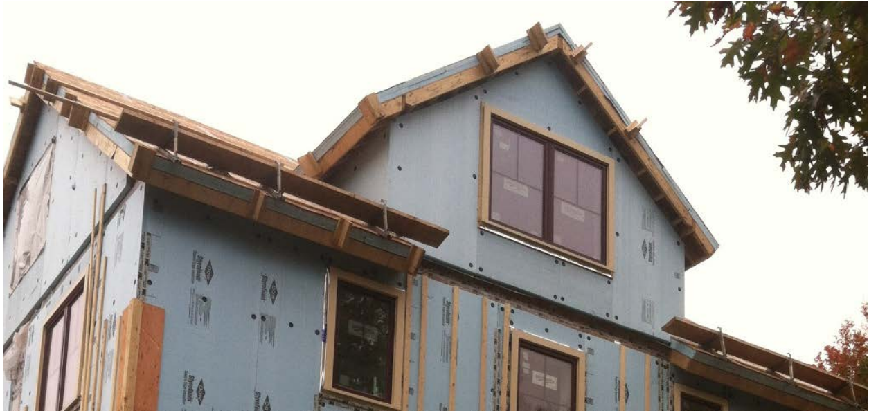
Figure 10. Four inches of XPS were installed above the first roof deck. A second deck, paper, and asphalt roofing were installed above the foam.
