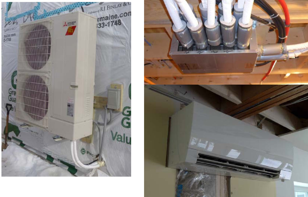
Figure 13. The heat pump outdoor unit in this BBH home under construction connects through a branch box to five ductless fan coils.
