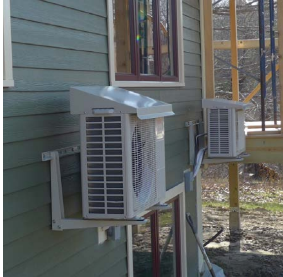
Figure 15. To ensure better winter performance, heat pumps are located well above snow level and covered to protect them from snow and ice.
