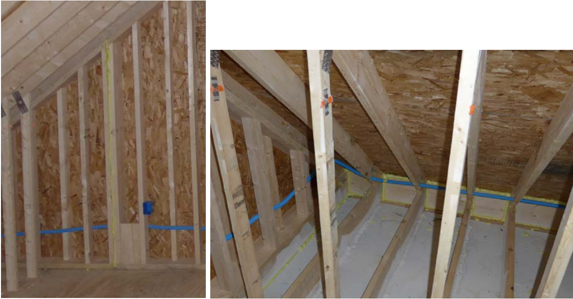
Figure 12. Gable wall and roof gaps appeared well sealed with foam and blocking.
