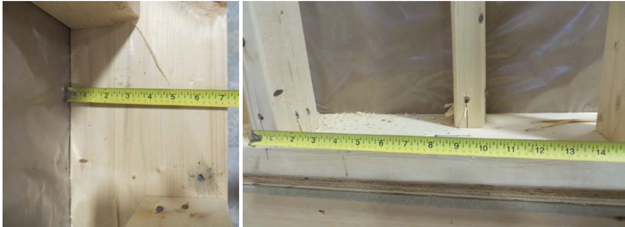
Figure 3. A 2x8 bottom plate with staggered 2x4 studs in the factory. The gypsum board is visible through the vapor retarder.
