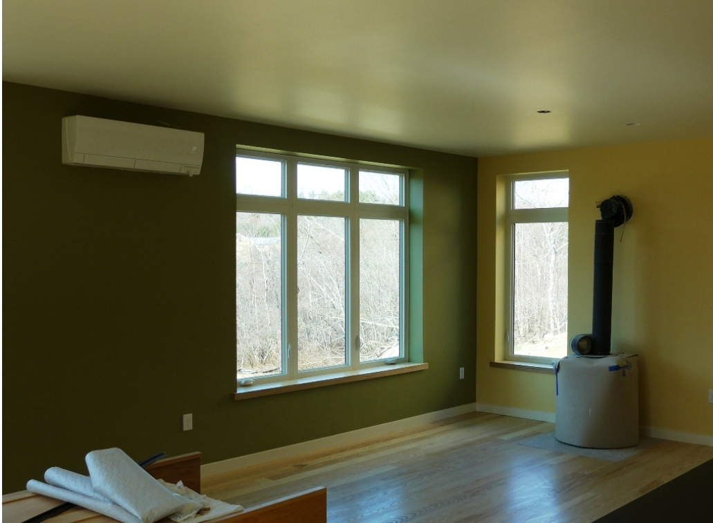
Figure 16. First-floor heat pump fan coil and wood stove
