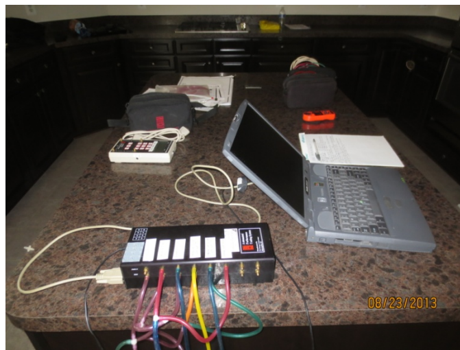
Figure 6. Six channels of pressure monitoring, using Energy Conservatory digital pressure gauge having auto ranging resolution of 0.1 Pa and accuracy of \pm 1\% of reading or 2 times the resolution, whichever is greater
