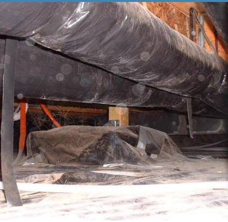
Artistic Homes followed Building America's recommendation to locate ducts in conditioned space to further the energy savings
