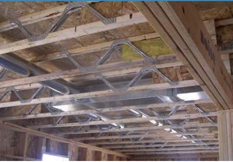
Open web trusses provide convenient paths for duct chases between floors in conditioned space
