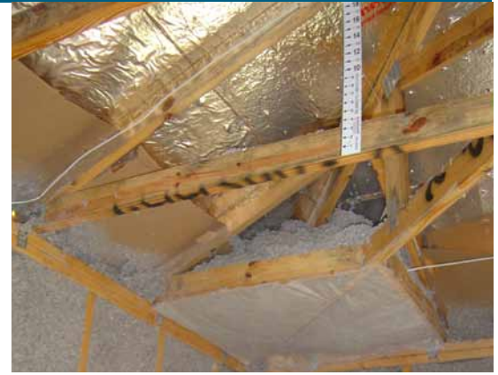
The walls and ceilings are insulated with naturally bug-resistant GreenFiber blown-in cellulose insulation – R-13 in the ceiling and R-30 in the walls. Note the special attention to insulating the corners. Also note radiant barrier installed along roof to minimize solar heat gain through roof.
