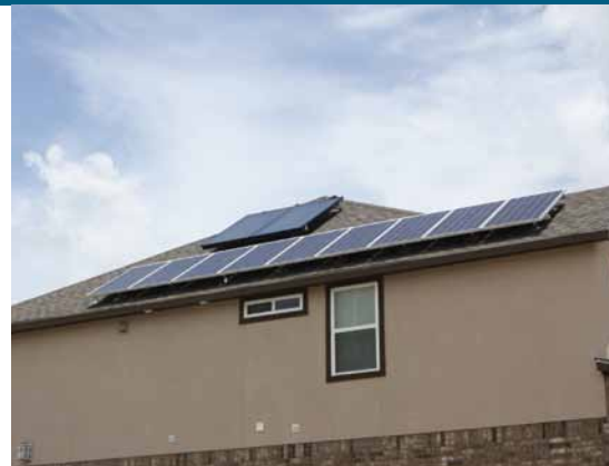
The Monterrey home features a thermal solar water heater expected to reduce energy use by 2,465 kWh annually.
