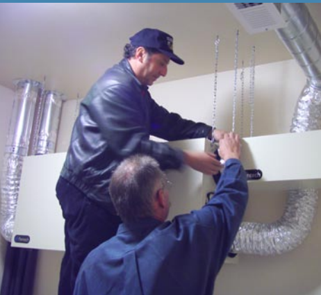
A Washington State University researcher and the construction manager install a monitor on heat recovery ventilation equipment.
