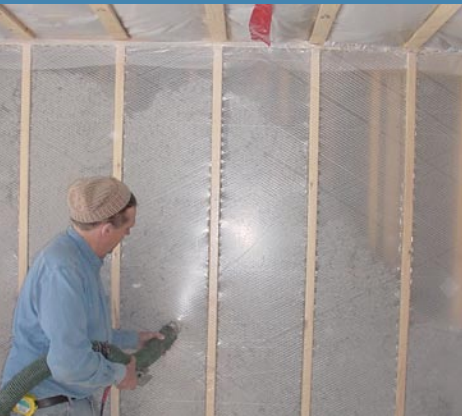
Double-stud walls contained over 11" of blown dry pack cellulose insulation to provide R-43 of wall insulation and an extra thick building envelope
