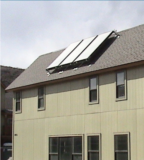
Solar water heating panels were mounted on each multifamily building to provide domestic hot water and pre-heat water for the hydronic baseboard space heating system.
