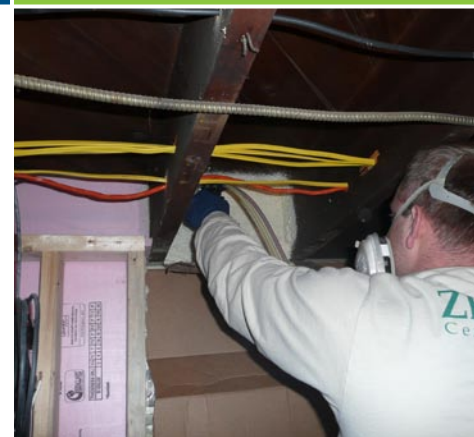
Spray foam was applied around piping and wiring holes and around pieces of rigid foam fitted in the rim joists
