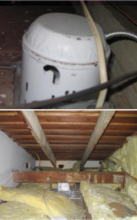
(top) Holes in 52 can (recessed) lights caused significant air leakage.
