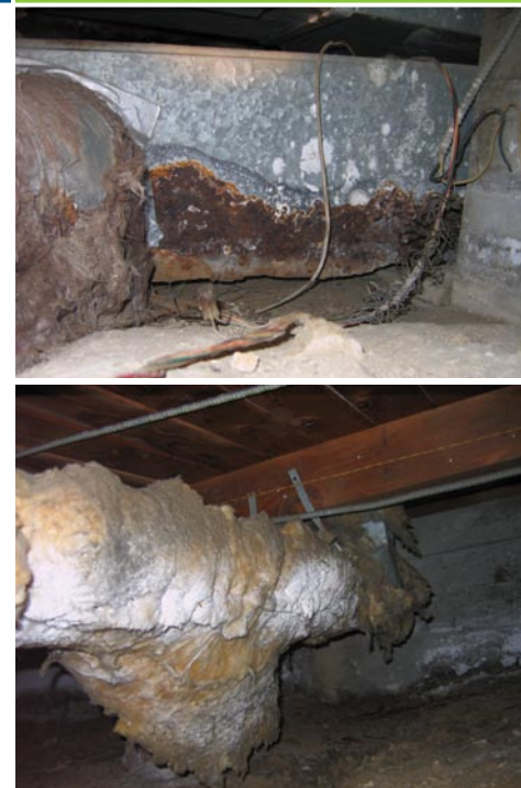
(top) The bottom of the furnace’s return plenum was completely rusted out.
