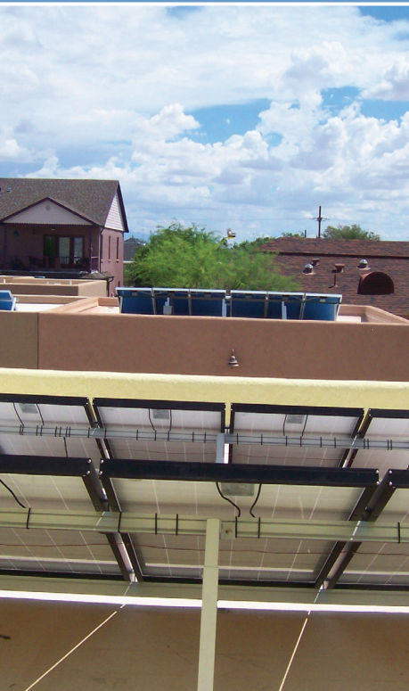
All homes come standard with a 1.5-kW photovoltaic system and solar hot water collector. (left) Photo courtesy of NAHBRC. (right) Photo courtesy of JWM.
