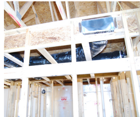
Artistic increases the efficiency of its heating and cooling systems by putting ducts in conditioned space in a central chaise down the main hallway.
