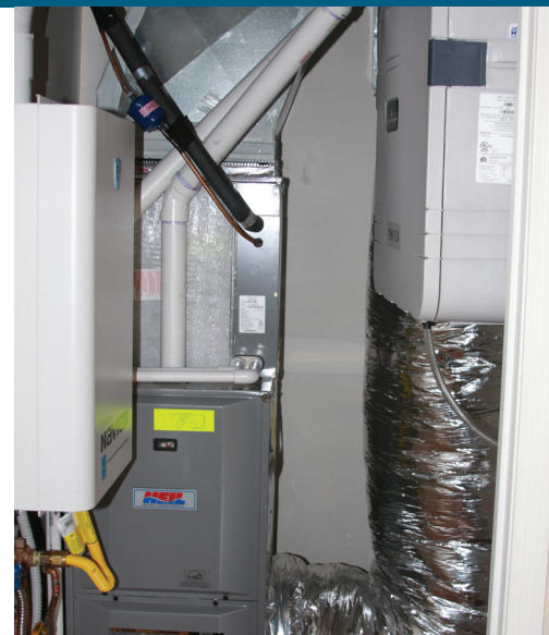
Artistic installs high-efficiency furnaces and ducts in conditioned space and provides a fresh air intake and heat recovery ventilator with HEPA filter for greater efficiency, air quality, and comfort.
