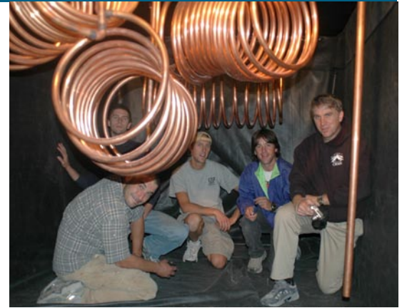
Eric Doub (right) kneels with other employees behind rolls of ¾-inch by 60-foot flex copper that serve as heat exchangers within the 6,000-gallon storage tank.
