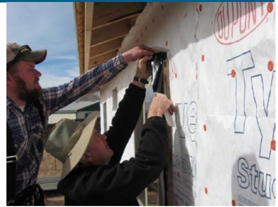
(photo at right) Yavapai College professor Tony Grahame and student Tommy Nester properly flash and install a window.
