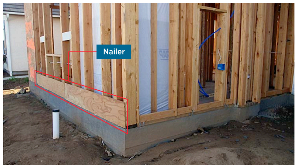
The slab edge of the test house prior to installation of the XPS rigid foam insulation, showing the nailer that supports the foam.
