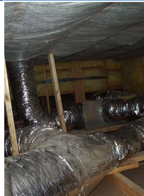
Ducts are located in conditioned space and mastic sealed to minimize heating and cooling losses.
