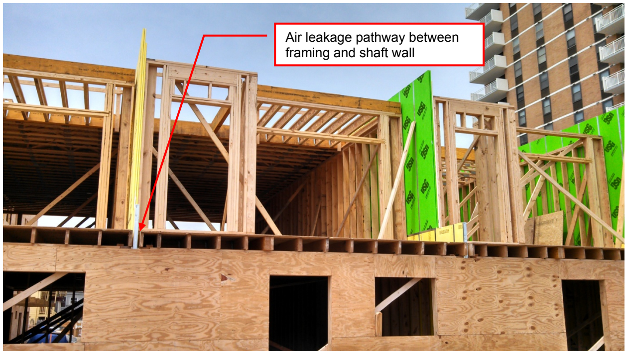
Figure 1. Fire separation walls (yellow or green gypsum shaft wall) in multifamily housing
