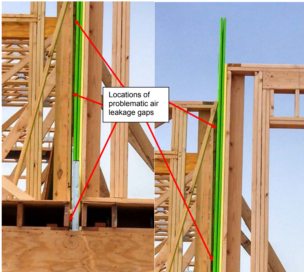
Figure 2. Examples of gaps where approved air sealing strategy is needed at the perimeter of fire separation walls
