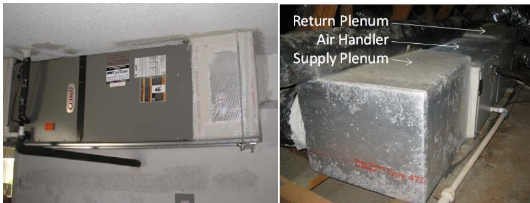
Figure 28. Horizontal flow AHUs mounted at ceiling of garage (left) and in the attic (right)
