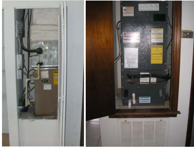
Figure 24. Upflow AHUs in conditioned space in a dedicated closet. Interior AHU closets with returns formed by platforms had wall-mounted return grilles with a full door on an adjacent wall (left) or a partial door above (right).
