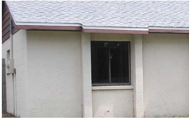
Figure 8. Typical wall construction of light color paint on stucco finish over concrete block
