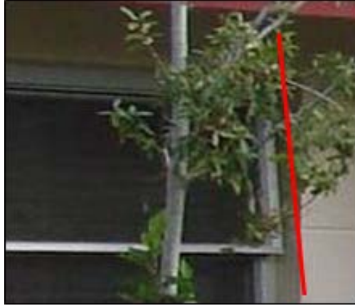
Figure 10. Pre-retrofit awning window in its most closed position is still slightly open, as indicated by the pitch of the red line.
