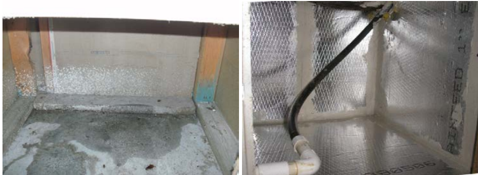
Figure 25. Return plenums were formed by either unfinished, open framing (left) or sealed duct board (right) or drywall.
