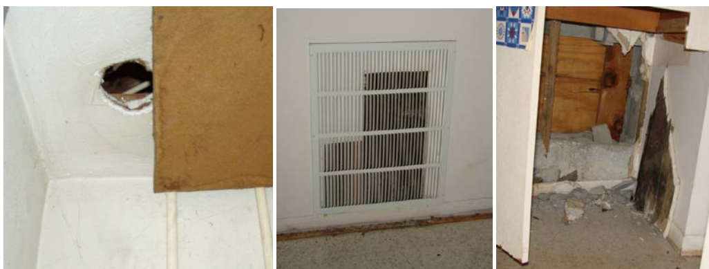
Figure 16. Pre-retrofit drywall penetrations: The ceiling fixture was removed, but penetration to the attic was unsealed (left); plumbing access in the wall covered with a return grille rather than a solid cover or patch (center); large opening beneath the bathroom vanity where block and drywall were removed as part of an incomplete renovation (right).
