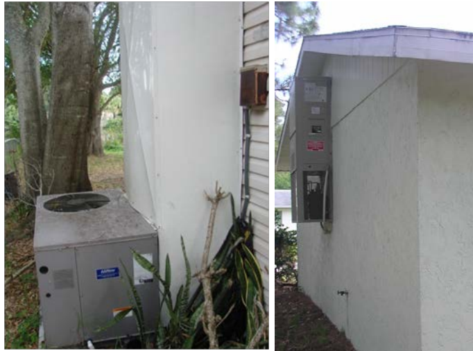
Figure 29. Exterior package units with return air path through a wall-mounted filter-back grille. Ground mounted unit with metal shroud housing main return and supply ducts (left) and wall-hung unit with attic-mounted ducts (right).
