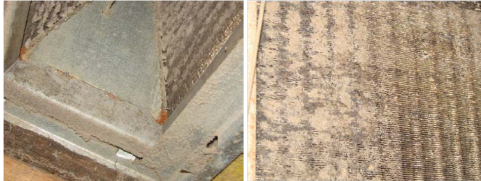
Figure 19. Looking up at pre-retrofit clogged, dirty cooling coils in the AHU (left); corroded and clogged cooling coil (right)
