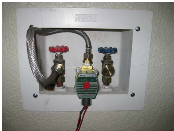
Figure 37. Water draw configuration in laundry closet
