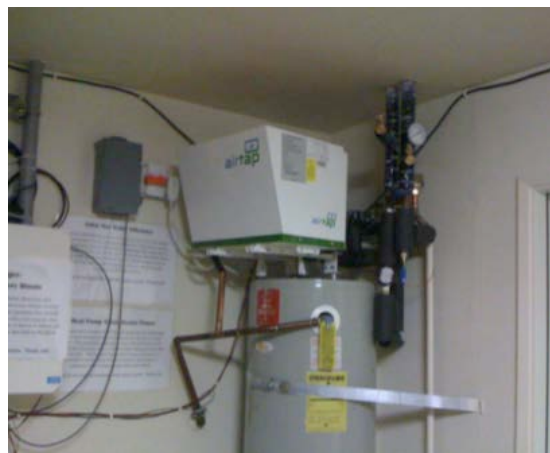
Figure 35. AirTap add-on HPWH NREL/PIX 19618, Credit: Lieko Earle
