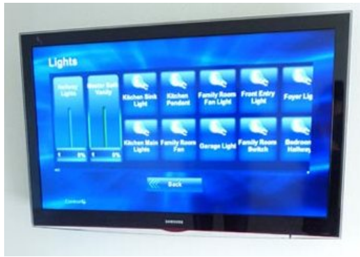
Figure 17. Control4 lighting control interface through the television
