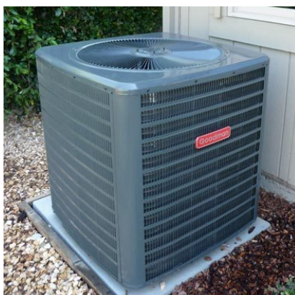
(b) High efficiency SEER 16, HSPF 9.75 heat pump (condenser unit) Credit: Judy Lew-Loose, SMUD
