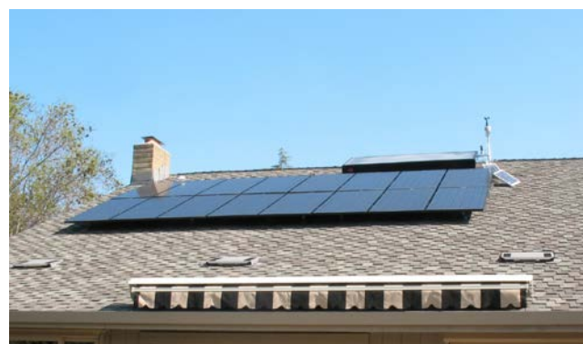
(b) The 2.3 kW PV array and the ISC SWH. Also shown is the weather station installed by NREL. NREL/PIX 19615, Credit: Lieko Earle
