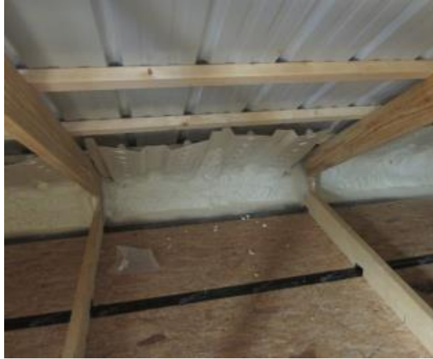
Figure 7. ccSPF installed over the outer edge of the double wall to the desired R-value for the ceiling
