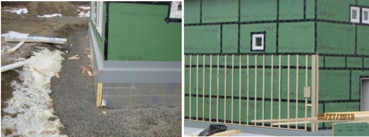
Figure 8. Flashing over slab edge insulation was taped to the sheathing using the manufacturer’s approved tape. The vented cladding was then attached with ¾-in. furring strips, and it overlapped the flashing.
