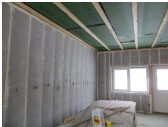
Figure 4. Full-depth cellulose insulation in a 12-in. double wall
