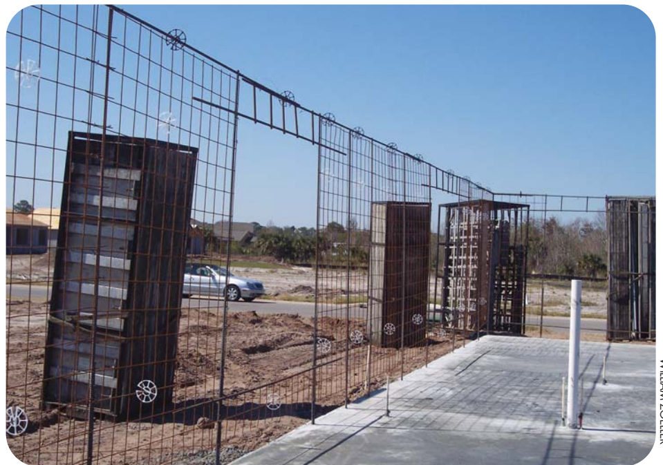
Mercedes Homes' concrete wall system starts with a steel-reinforcing cage consisting of a 6 x 6 steel mesh and vertical #5 steel bars placed at 48 inches on-center.
