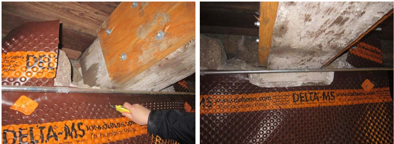
Figure 23. Air gap membrane venting to underside of beam (L); retrofitted detail (R)
