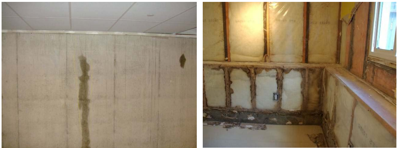
Figure 1. Active seepage through cast concrete (L); water damage concealed behind finishes (R)
