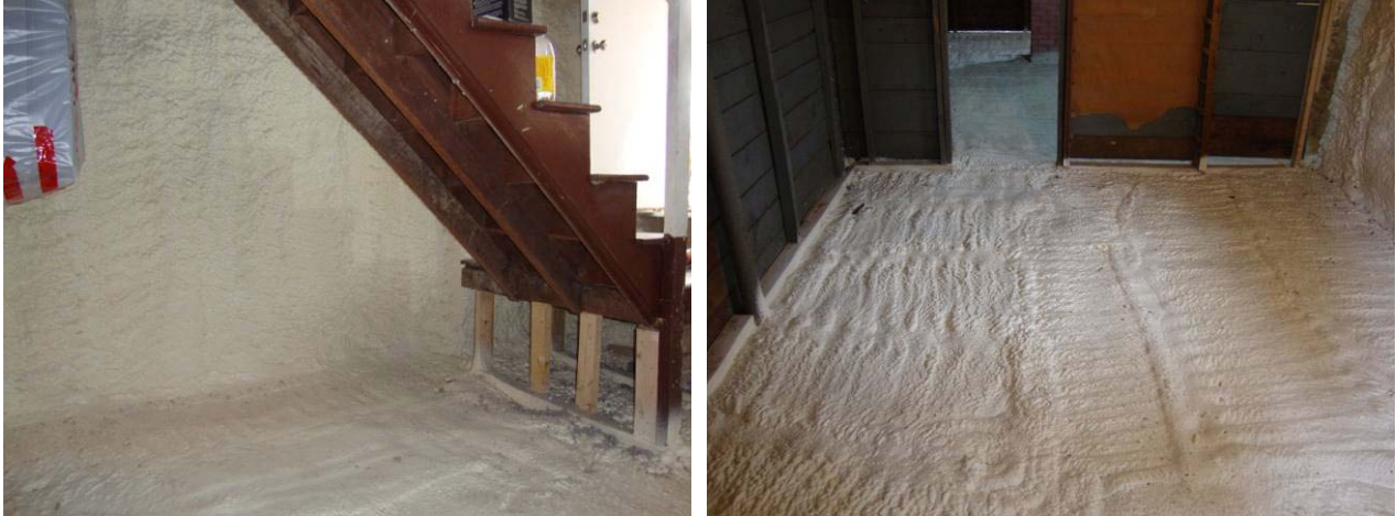
Figure 33. Spray foam applied to walls and slab (© 2011 by Byggmeister; reprinted with permission)
