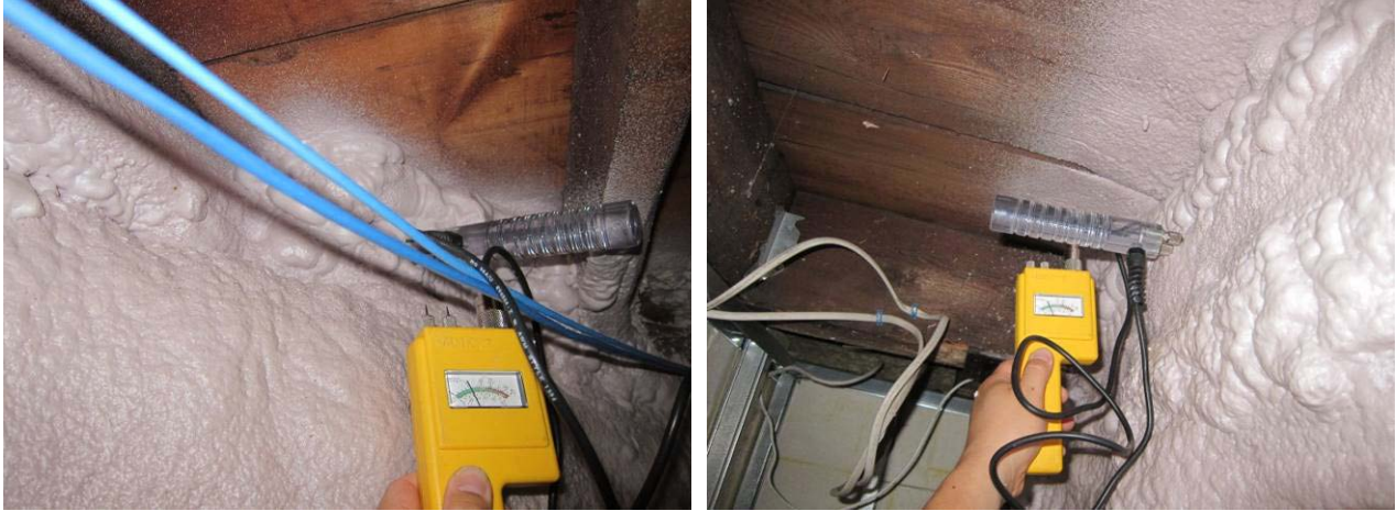
Figure 59. Sill beam moisture content measurement, Somerville Office
