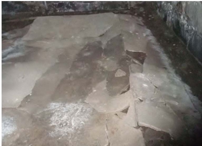
Figure 9. Basement slab heaving in unheated basement (Lstiburek 2010b)
