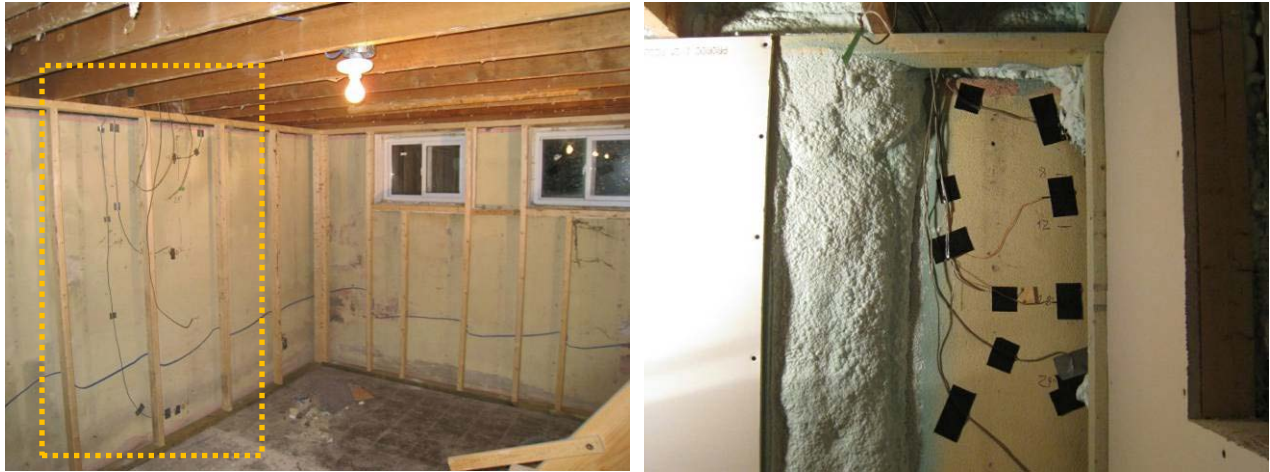
Figure 62. Overview and close-up of instrumentation in ccSPF retrofit basement
