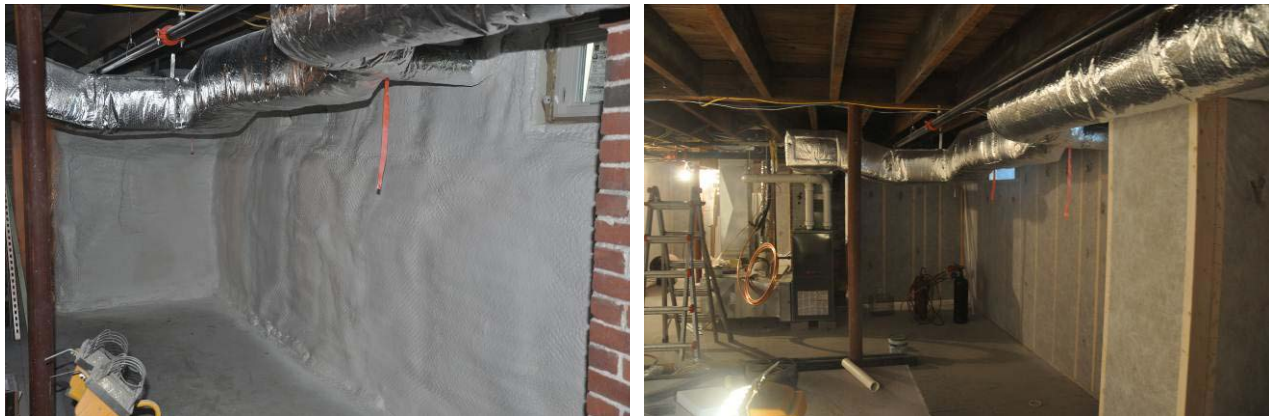
Figure 25. Basement with spray foam (L); and added cellulose in framed wall (R)
