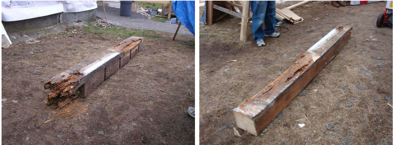
Figure 43. Damaged sill beams from Bedford Farmhouse
