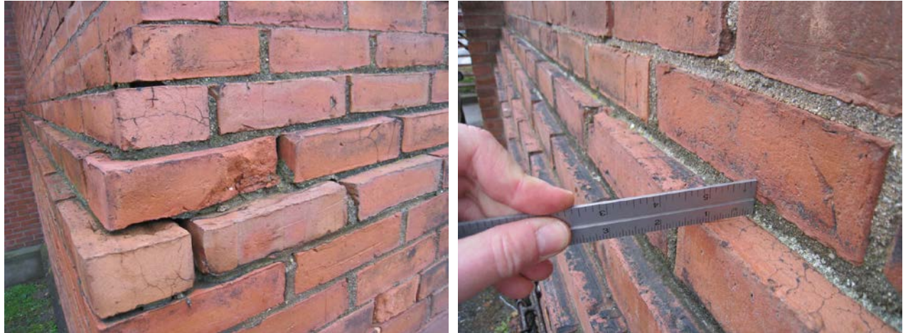
Figure 50. Steps in brickwork, and related cracking/FT damage
