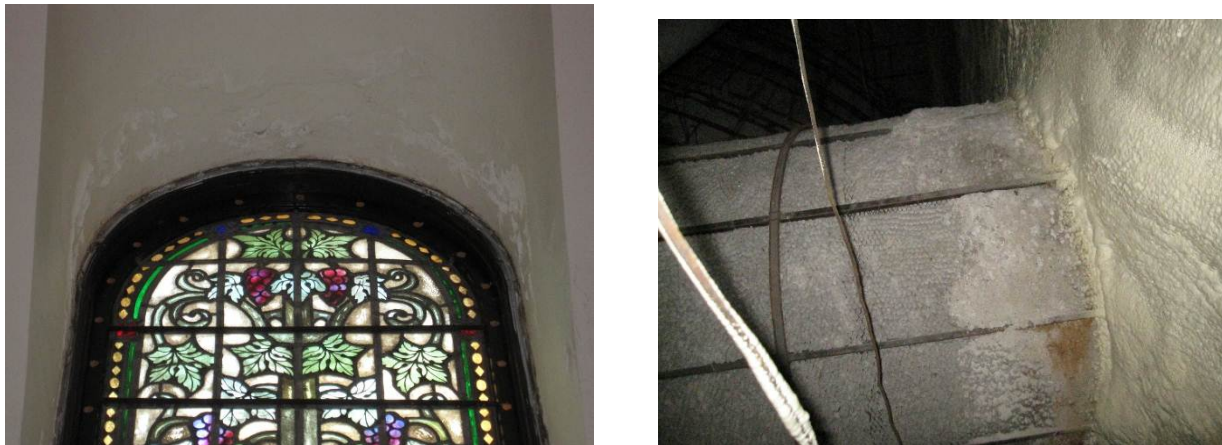
Figure 58. Moisture issues at chapel windows
