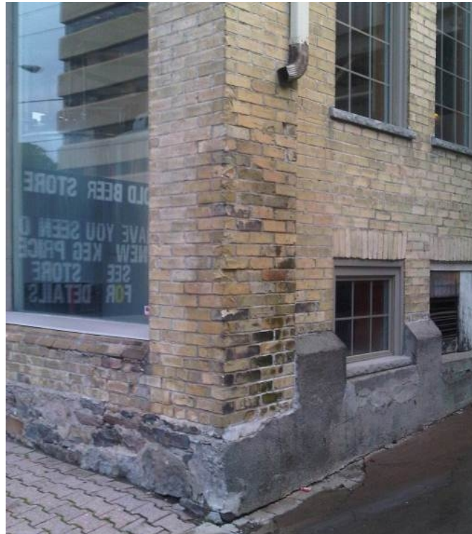
Figure 66. Disconnected downspout and related damage to masonry
