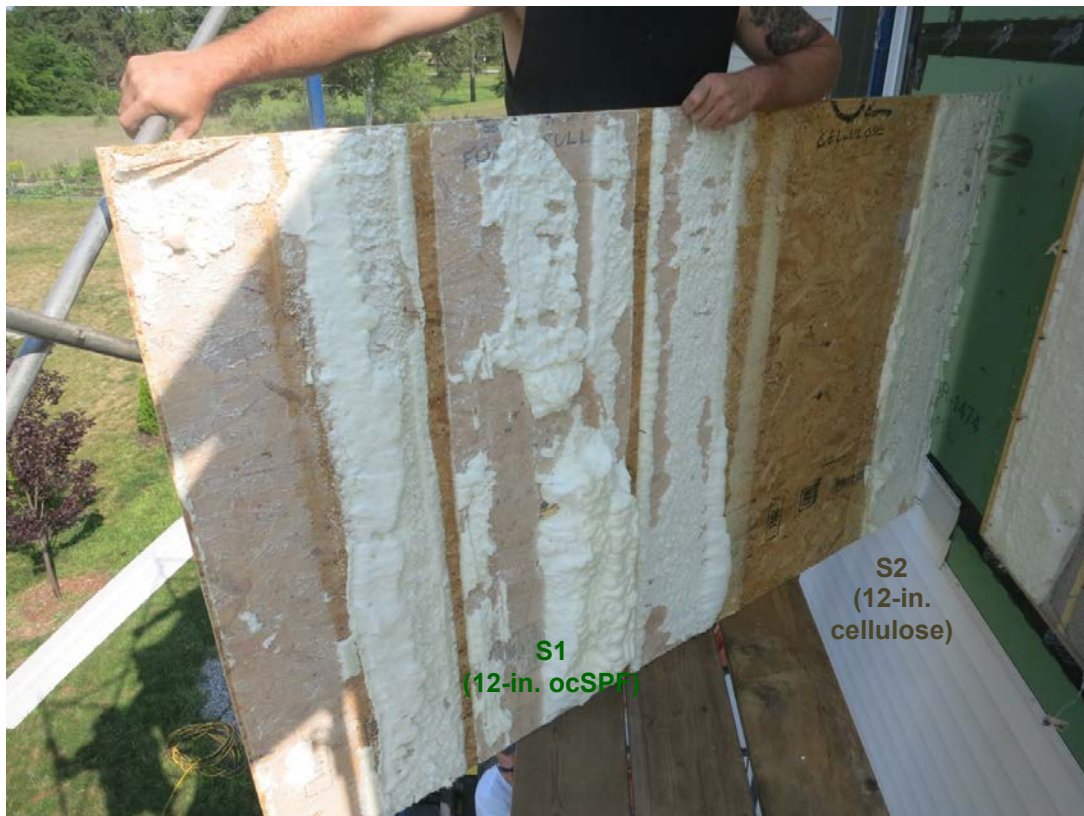
Figure 40. South-facing wall sheathing conditions
