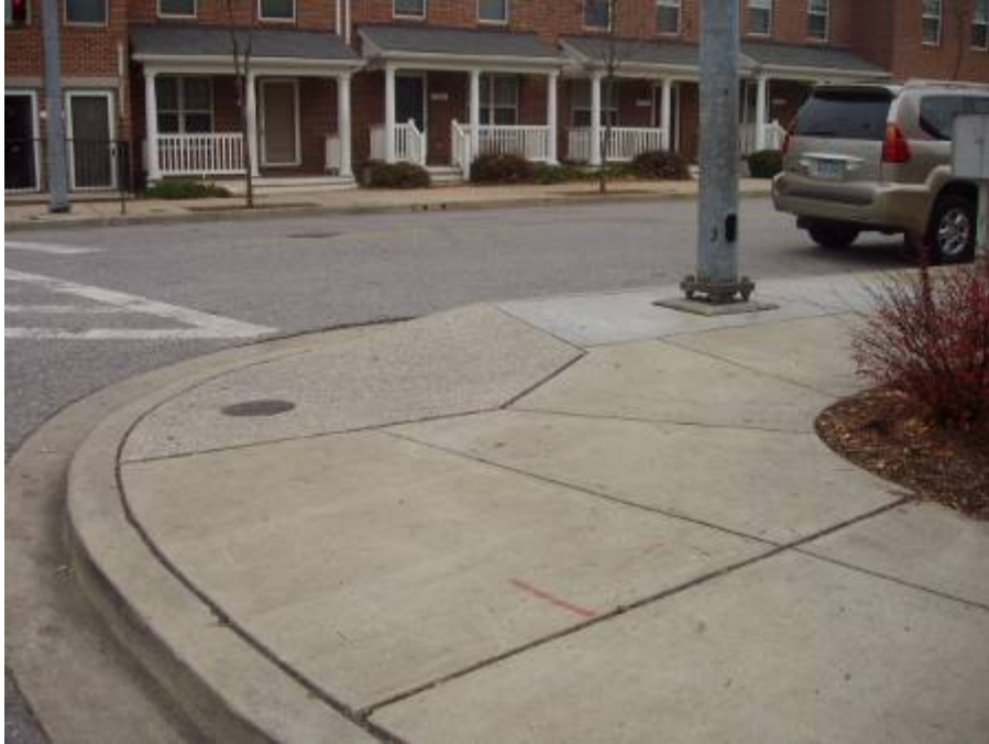
The accessible route is brought around the top of the curb ramp slope.
