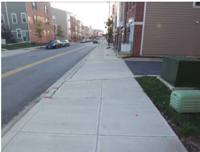
The picture at left demonstrates the excessive cross slope of the route as it negotiates across the driveway.
