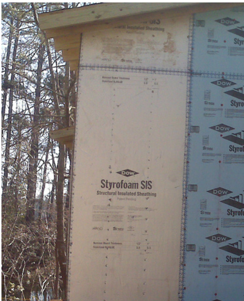
Framing is covered with XPS foam structural insulated sheathing instead of OSB. The foam sheathing provides R-3 of insulation and protection against moisture. The wall cavities are filled with an additional R-13 low-density spray foam insulation, which provides air sealing as well as insulation.
