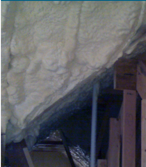
Unvented attics insulated with R-30 low-density spray foam provide a semi-conditioned space for the high-efficiency heat pump and ducts.
