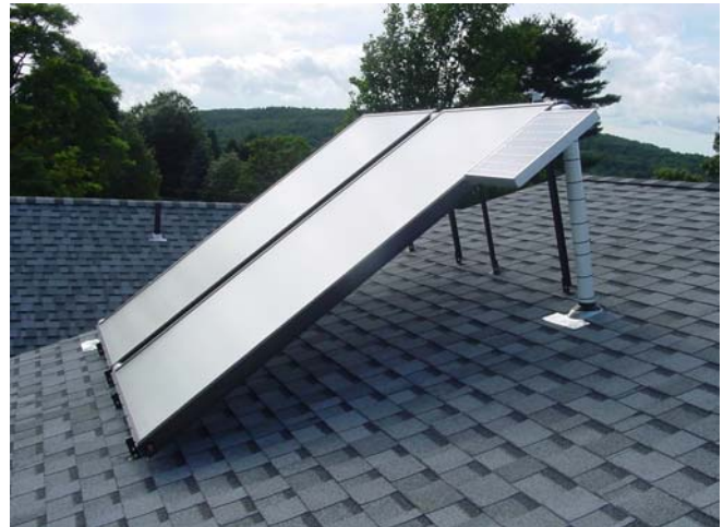
Fig. 1: Roof top solar collectors on the Massachusetts home.
