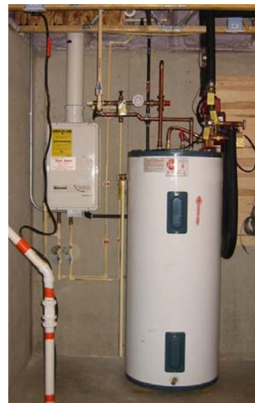
Fig. 3: Auxiliary tankless gas water heater and solar storage tank in basement of Madison home.
