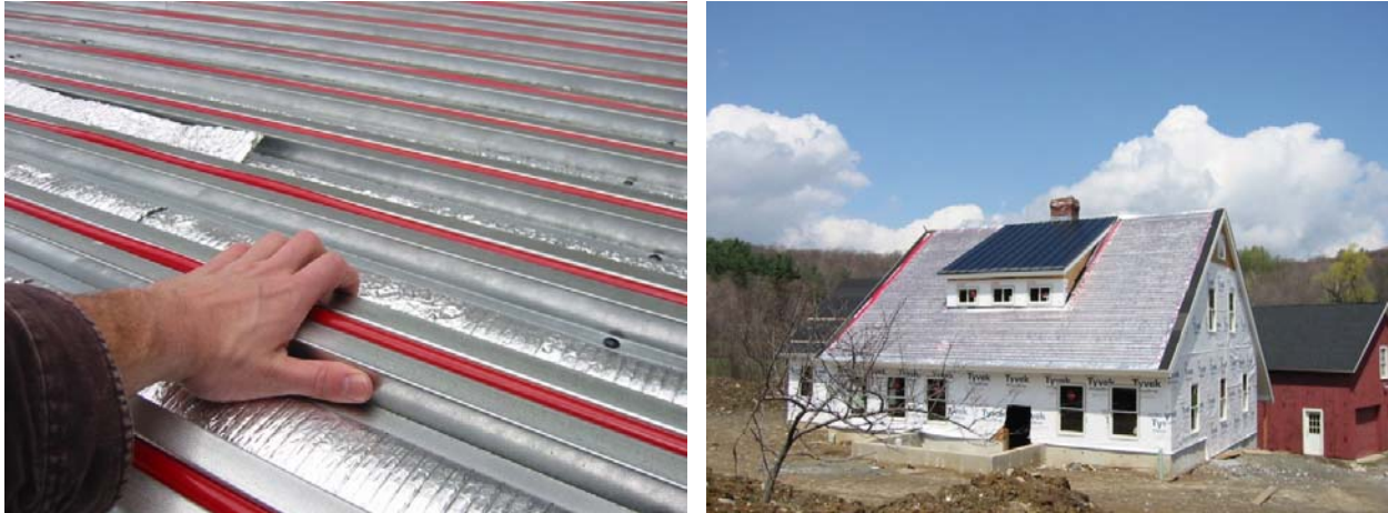
Figure 2. The home during construction. Solar thermal and PV collectors have been installed on the shed dormer. Metal roofing has not yet been installed over PEX tubing and heat transfer purlins on the main roof area.
