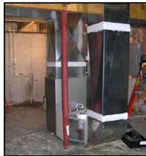
Mastic coating the Supply/Return trunks
