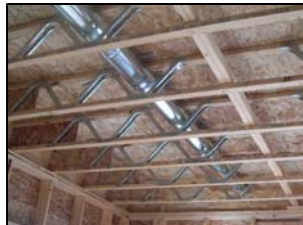
Integrated HVAC System
