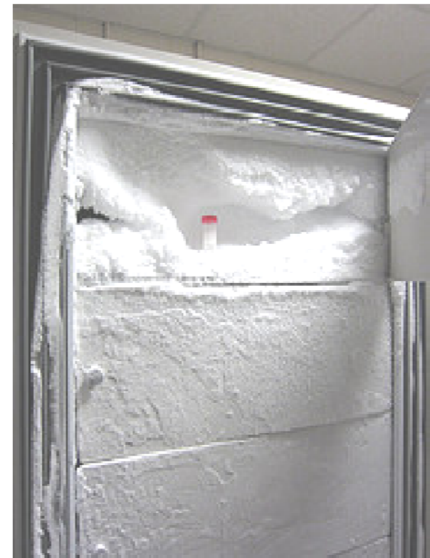
Frost buildup caused by inadequate maintenance. Photo source: UC Davis
