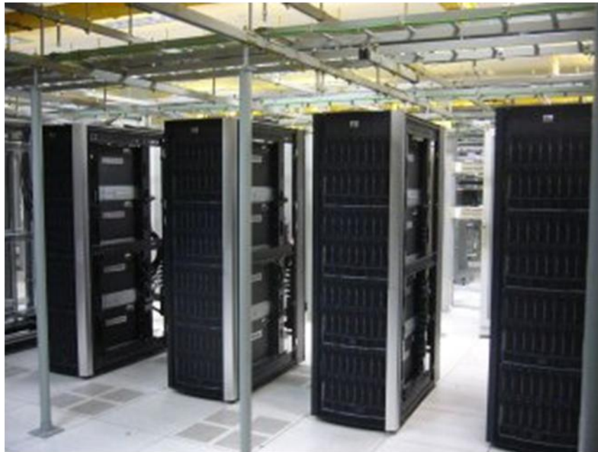
Figure 5-4: Server Racks in a Data Center
