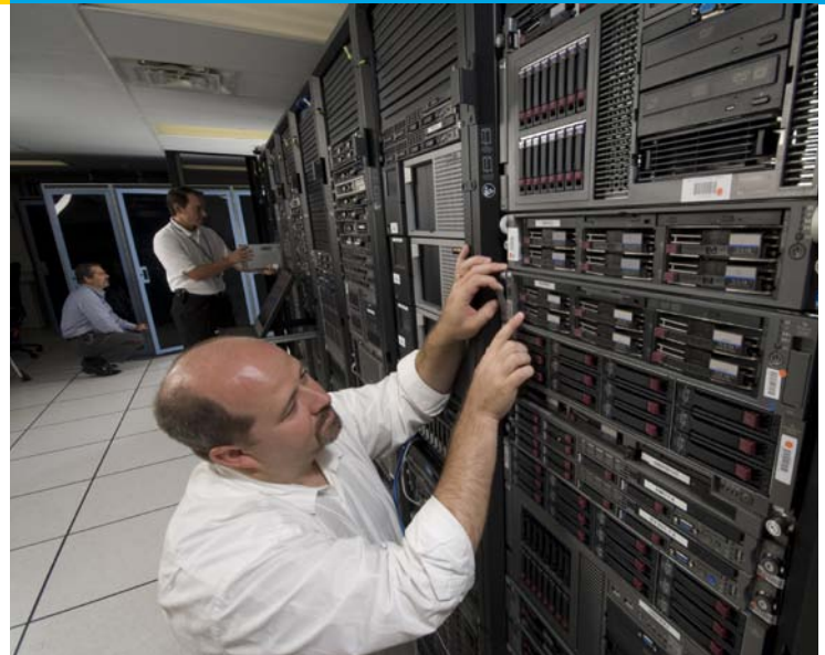
Figure 1. NREL's legacy data center
