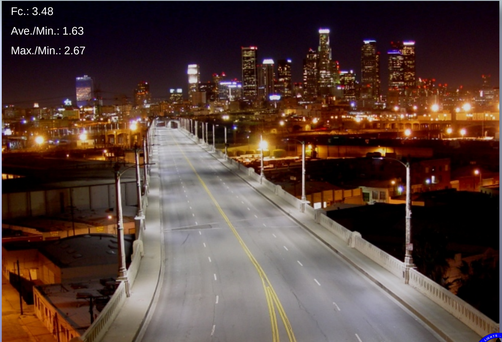
AFTER – 180 W LED (180 W) 6th Street Bridge over Los Angeles River
