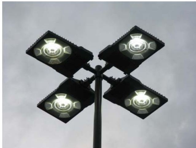
Figure 2.8. GE luminaires on top of poles
