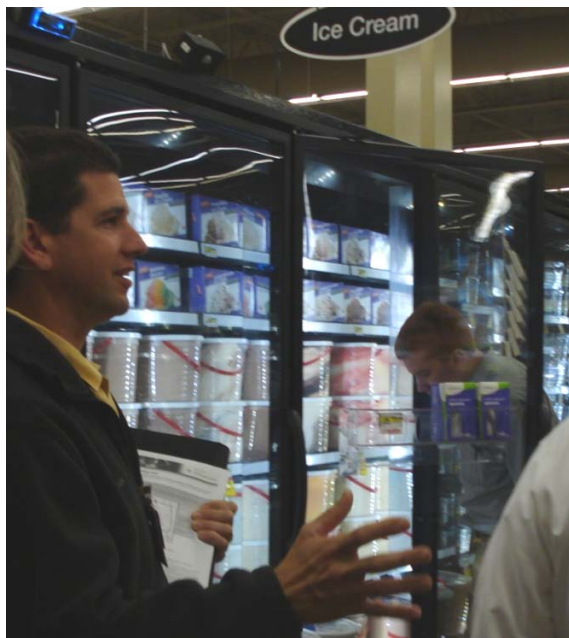
Frozen food cases sport LED lighting and motion sensors that dim to 20% output when the aisle is unoccupied.
