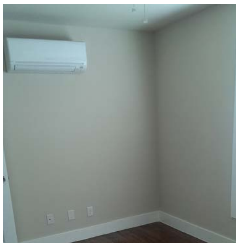
A high-performance ductless heat pump provides all of the home's heating and cooling.
