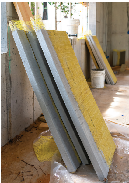
All of the exterior walls are wrapped in 2 inches of rigid mineral wool insulation.
